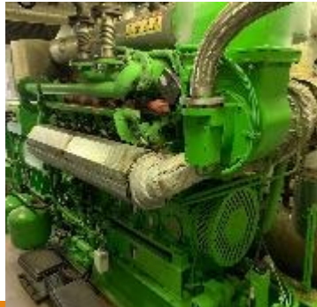
20 kW ORC / Biogas Germany 2020
