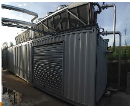
40 kW ORC / Landfill gas France 2015
