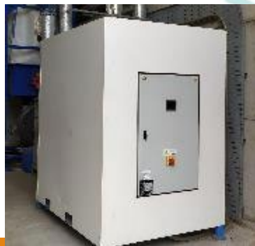
40 kW ORC / Biomass boiler UK 2018
