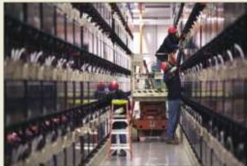
The world's largest battery energy storage system.
