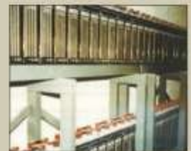
The battery energy storage
